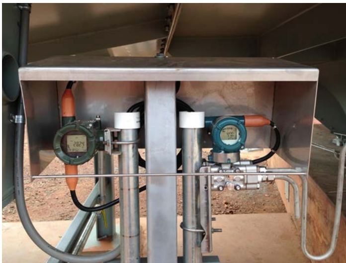
The shaft collar pressure and air temperature monitors transmit real time data with the ability to enable automatic calibration.
