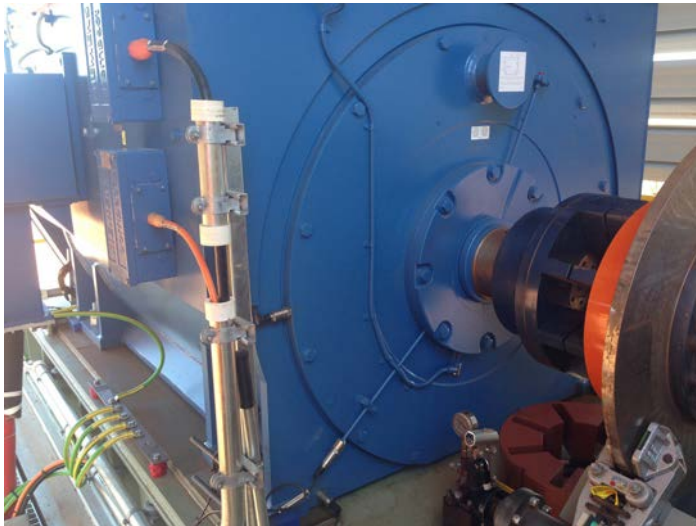
Motor vibration sensors attached to the fan measure vibration velocity, as well as monitor temperature and vibration levels.
