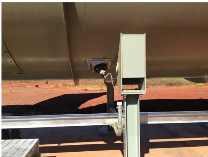
An Accutron flow sensor in the fan duct helps monitor, control, and diagnose potential problems with air flow.
